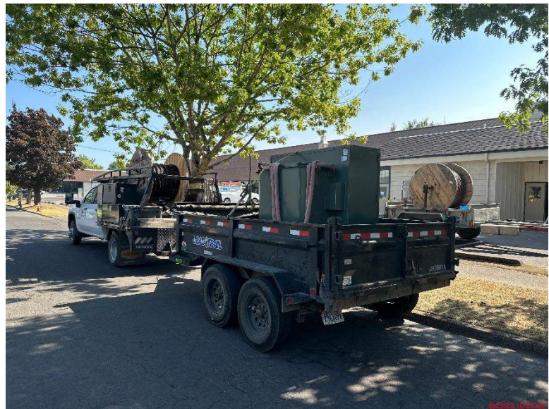
Cache Valley (PPL) Onsite 8-23 With New Transformer
