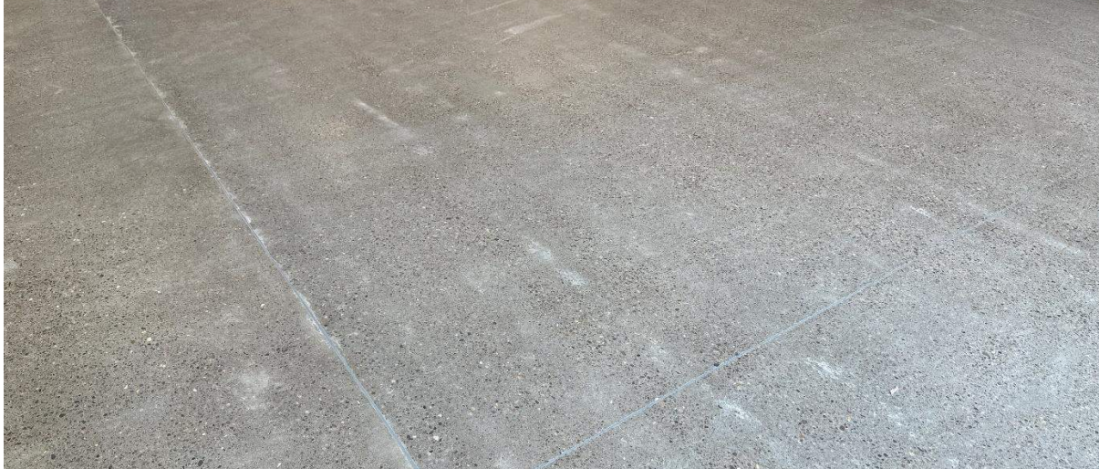
Poorly Polished Concrete - Rejected
