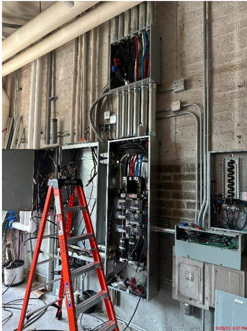
Electrical Room Before New PPL Service
