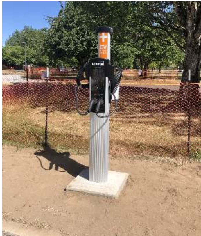
New EV charging station
