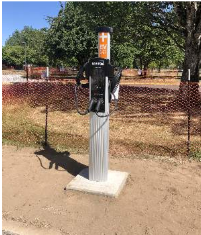
New EV charging station
