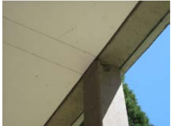
Figure A10.3.e – Cracks at exterior columns
