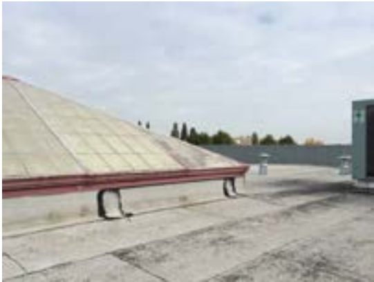
SKYLIGHT WEARING THROUGH
