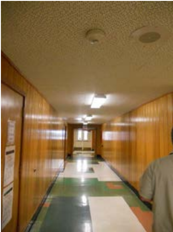
Figure D10.3.a – Hallway lighting
