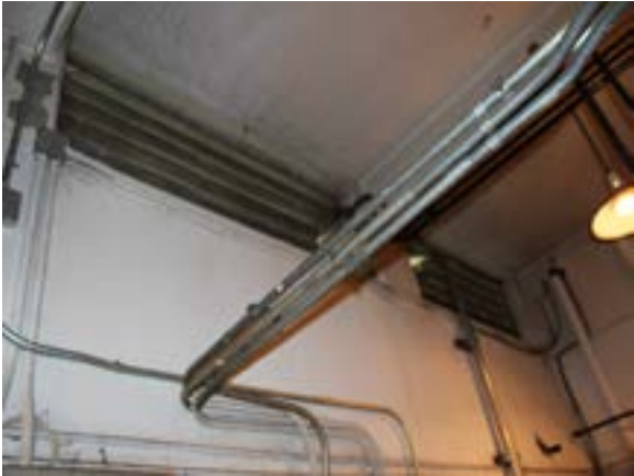
Figure D10.2.f – Conduits need additional support
