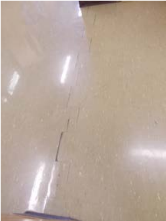
Figure B20.1 – Flooring issues
