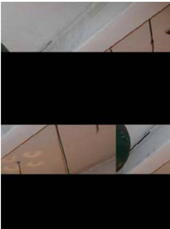
Figure D10.3.c – Mechanical room lighting
