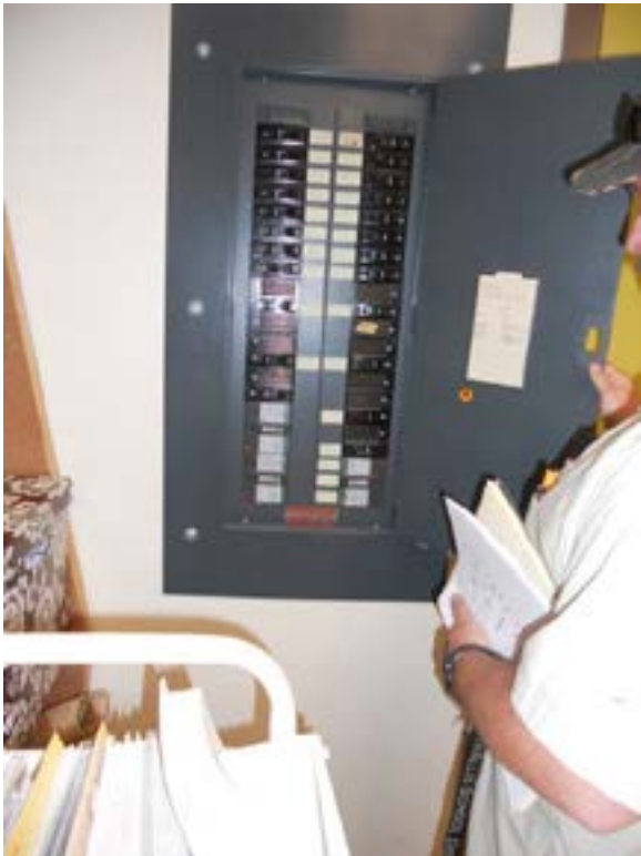
Figure D10.2.b – Lack of panel capacity
