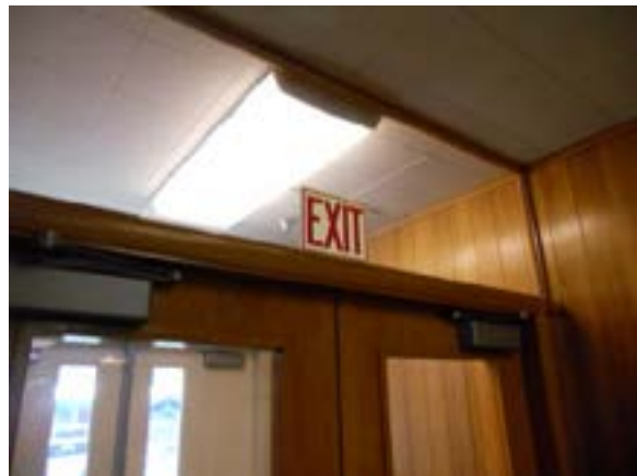
Figure D10.7 – Photoluminescent exit sign
