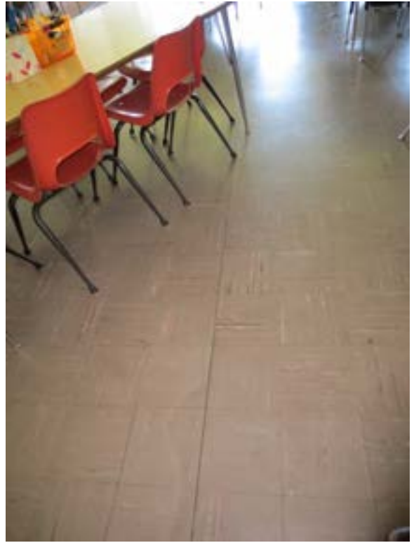
Figure A10.3 – Crack in Room 14 floor finish
