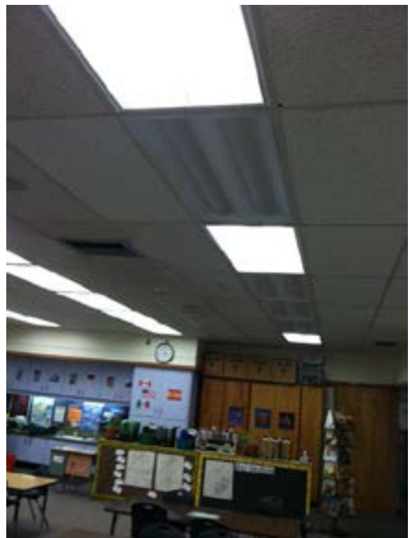
Figure D10.3.a – Typical ballast failure
