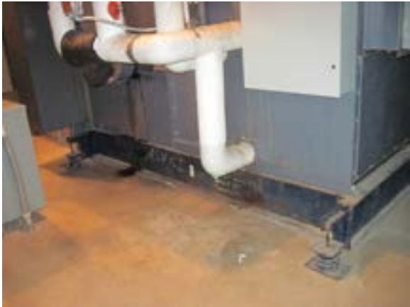
Figure A10.3.h – Equipment not anchored
