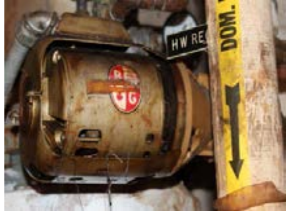
Figure C20.7.b – Hot water piping/pumps
