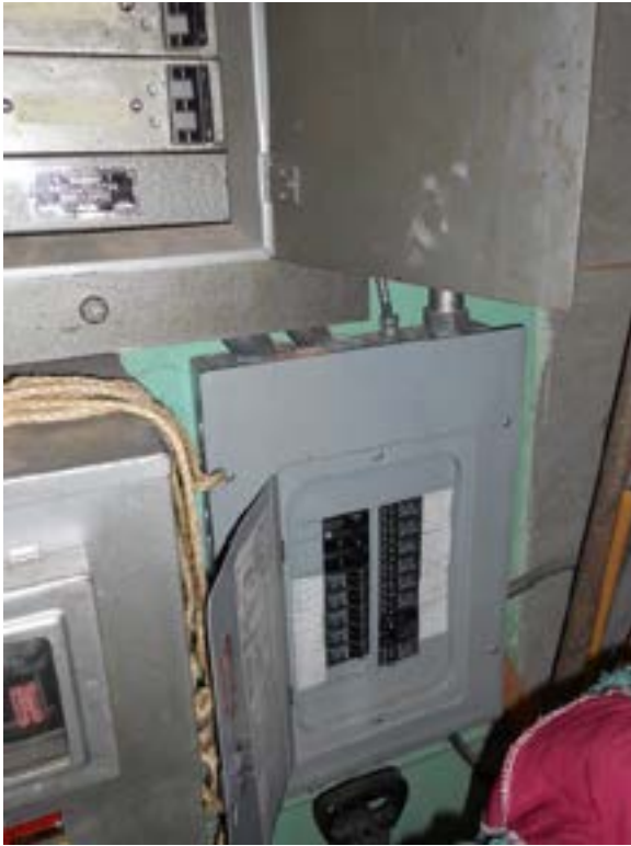
Figure D10.2.a – Panelboard with too many tandem breakers
