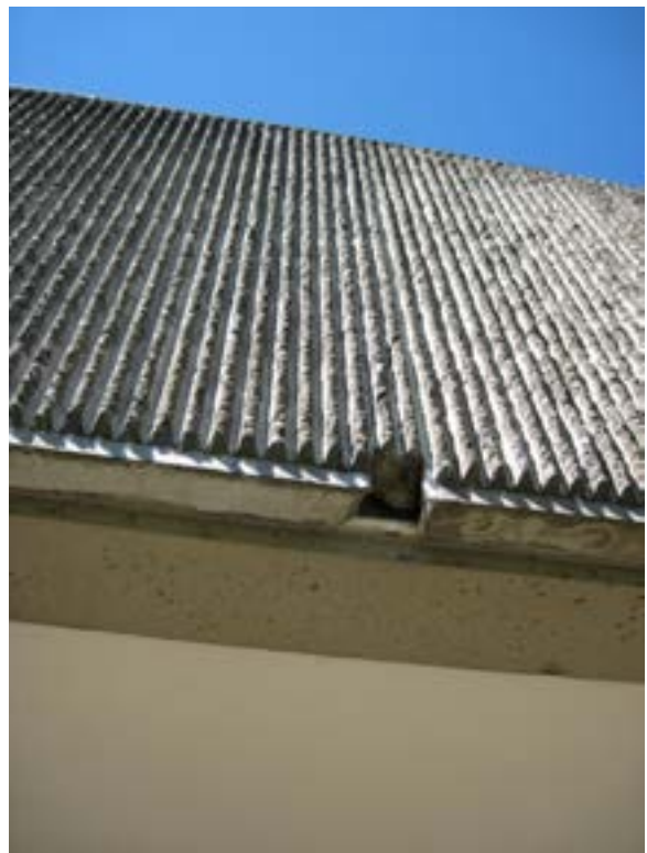
Figure A10.3.g – Fascia panel joint cracks
