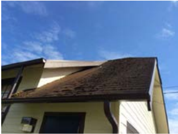
SHINGLES SHOULD HAVE MOSS REMOVED
