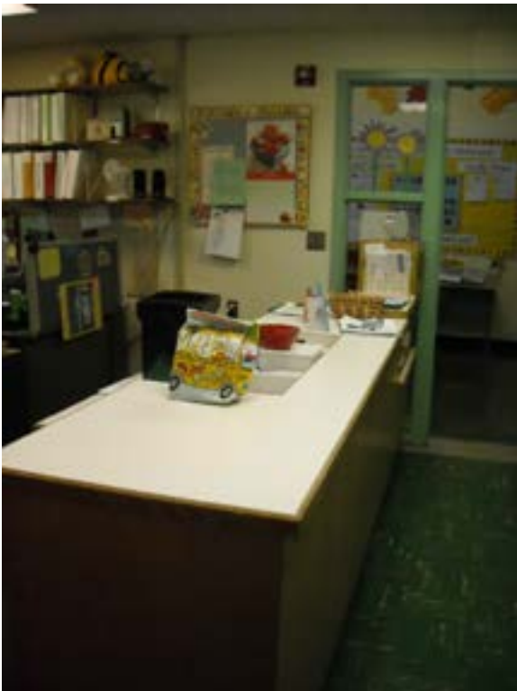
Figure B30.6 – Undersized main office
