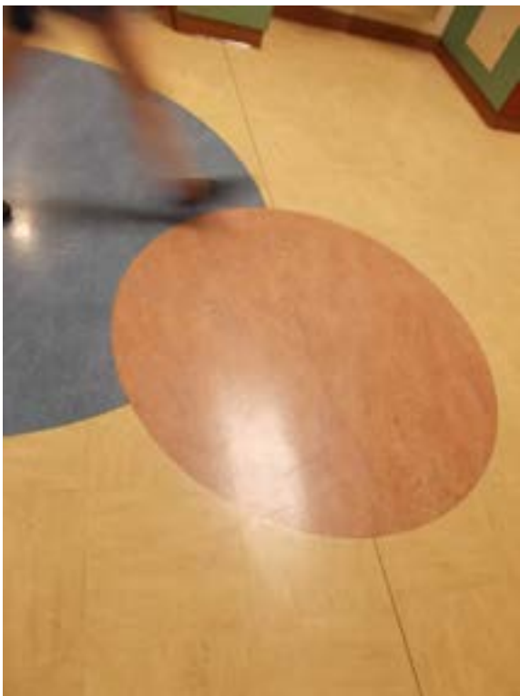
Figure B20.1.a – Flooring issues
