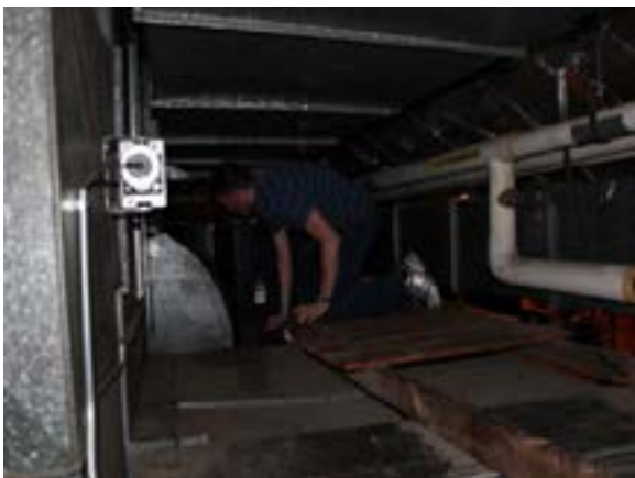
Figure C20.1.a – Poor equipment access
