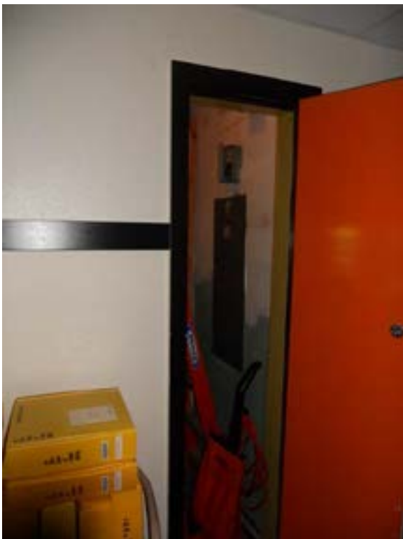
Figure D10.2.c – South electrical room
