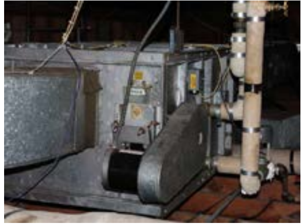
Figure C20.1.a – Forced air equipment
