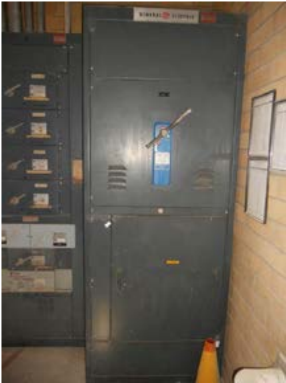
Figure D10.2.a – Pressure switch not maintained
