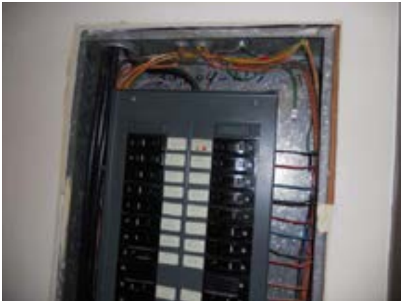
Figure D10.2.c – Grounding conductors missing
