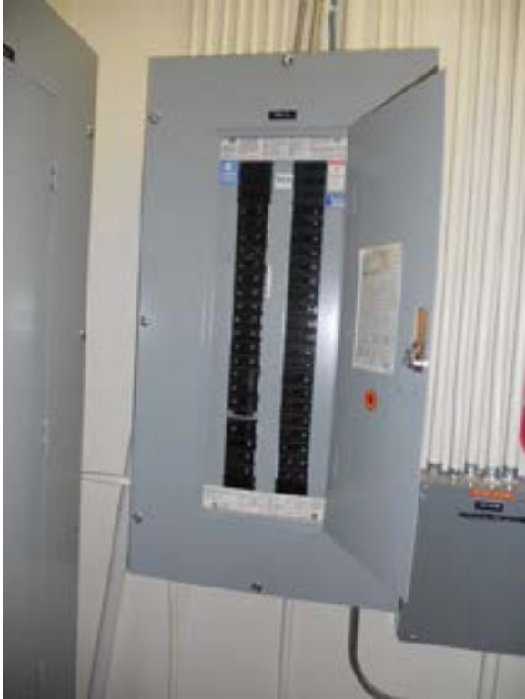
Figure D10.2 – Panelboard lacks capacity
