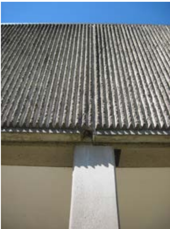
Figure A10.3.f – Fascia panel joint cracks
