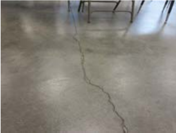
Figure A10.2a – Slab on grade cracking
