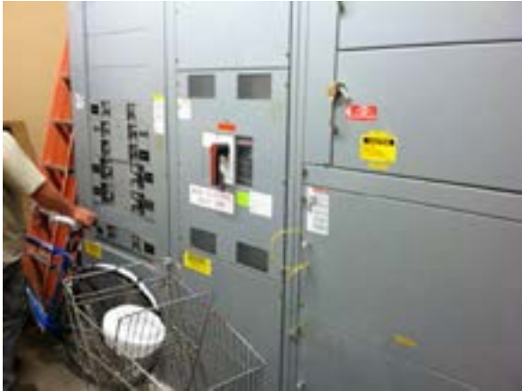
Figure D10.2 – Inaccessible switchboard
