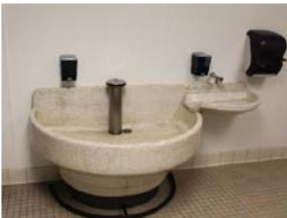
Figure C10.3 – Typical restroom fixture
