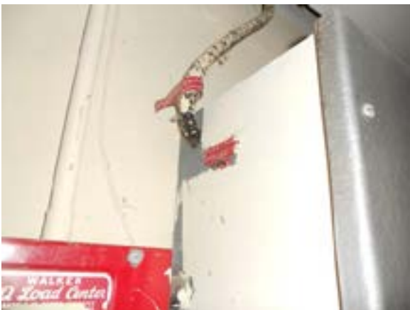
Figure D10.2.b – Conductor subject to damage
