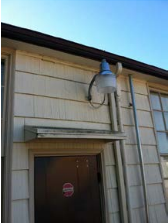
Figure D10.2.f – Armored cable used outdoors
