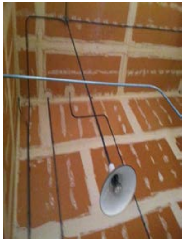
Figure D10.3.b - Failing lighting
