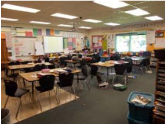
Figure B20.1.b – Flooring issues
