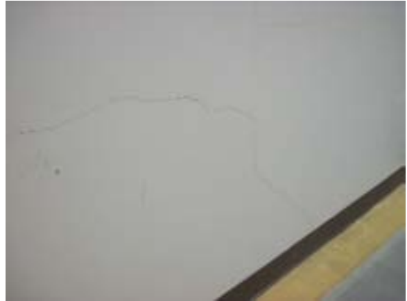
Figure A10.3.a – Cracks in panels
