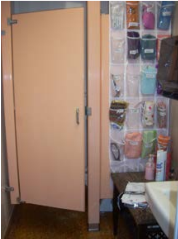
Figure D40.8 – Staff restroom
