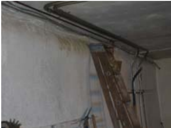
Figure A10.2 – Bulging plaster in boiler room
