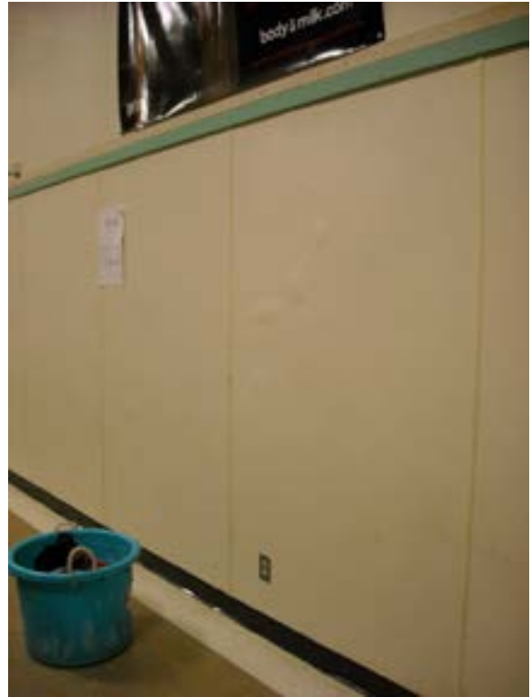
Figure B20.6 – FRP panels in cafeteria
