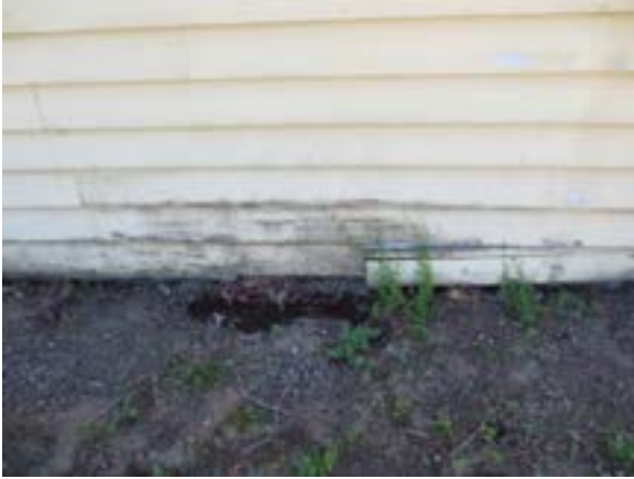
Figure A10.2 – Holes in crawl space
