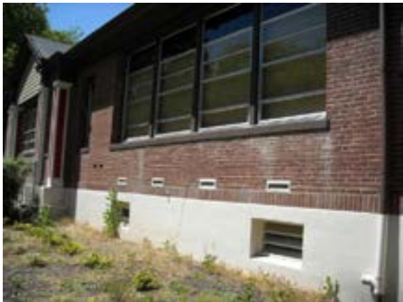
Figure A20.1 – Damaged concrete
