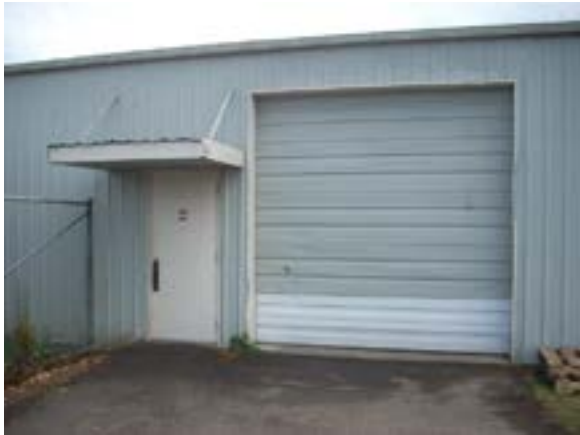
Figure A20.2.a – Rusted door
