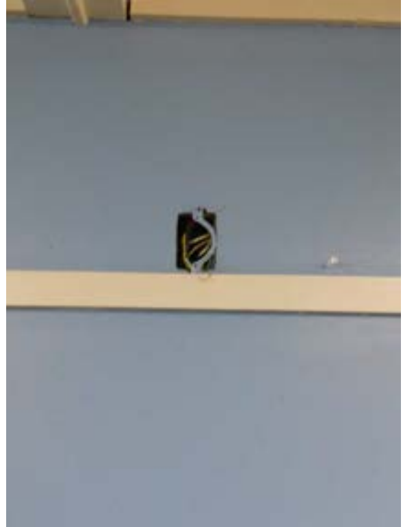
Figure D10.2.b – Junction box lacks cover
