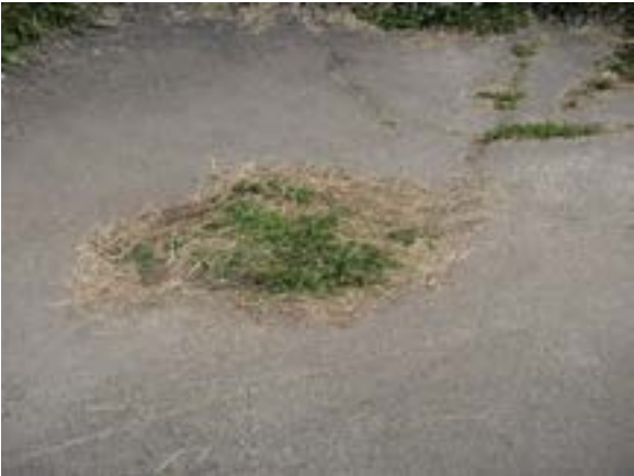
Figure E20.10 – Overgrown storm drains
