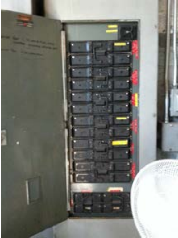
Figure D10.2.a – Main distribution panel
