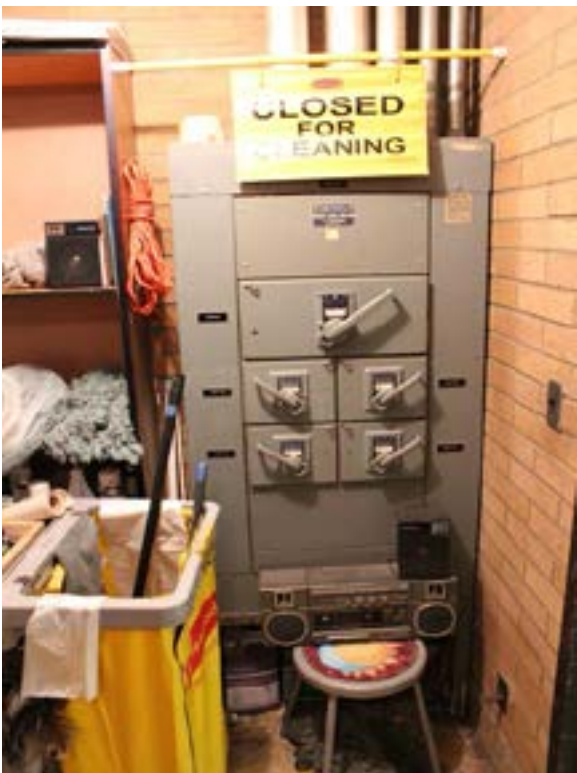
Figure D10.2.a – Blocked panel
