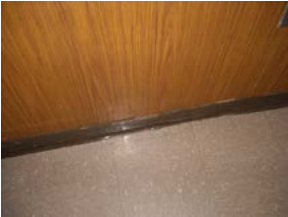
Figure B20.6 – Damaged base
