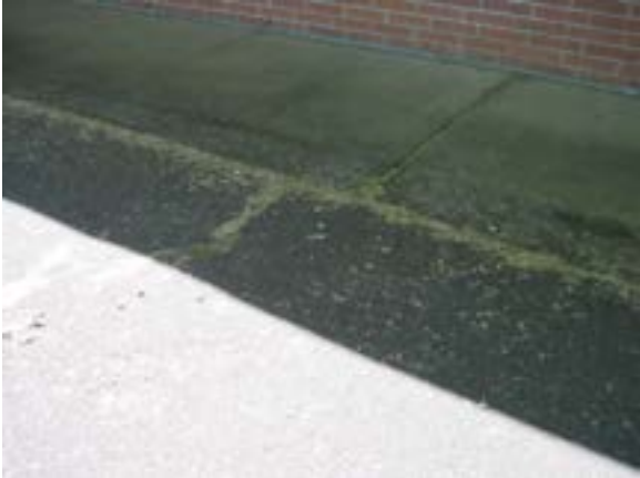
Figure A10.2.a - Ridge in slab/sidewalk
