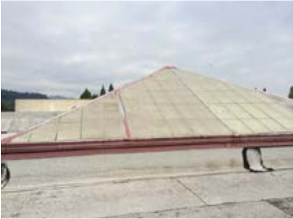
Fiberglass Skylight weathering through
