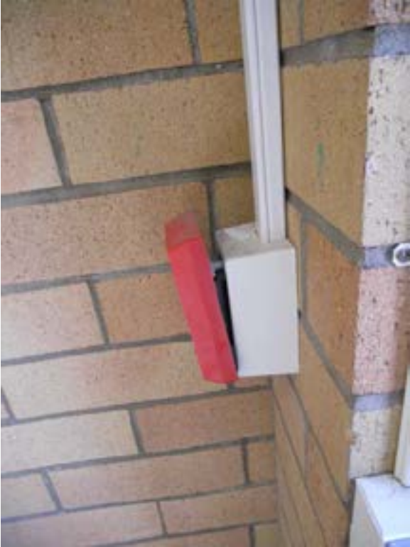
Figure D20.3 – Vandalized pull station
