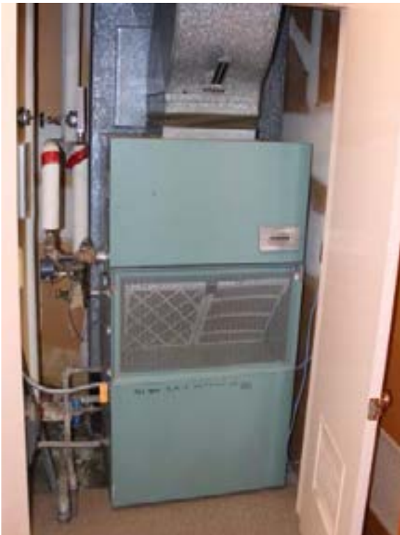
Figure C20.1.b – Library mechanical unit
