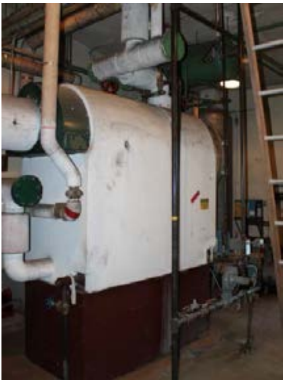
Figure C20.7 – Hot water boiler
