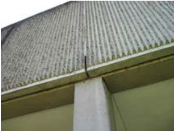
Figure A10.3.d – Cracks at exterior columns
