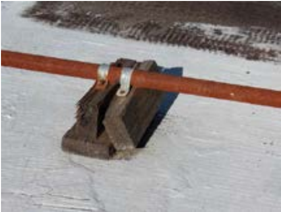
Figure C10.2 – Rusting pipes/rotted supports
