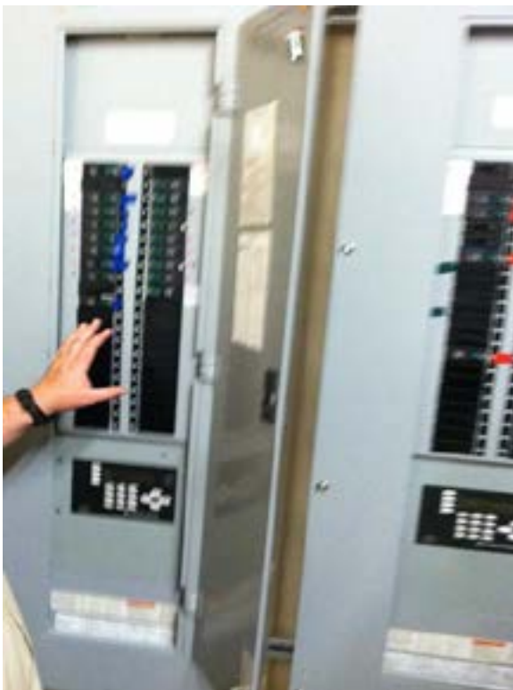
Figure D10.4 – Lighting control issues
