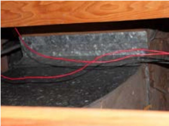
Figure D20.1 – Unsecured fire alarm wiring
