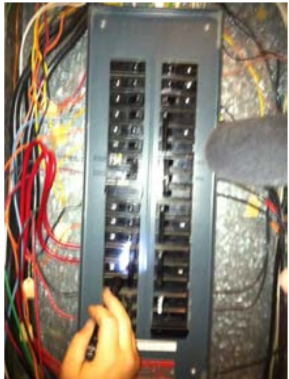
Figure D10.2.b – Grounding bus bar missing
