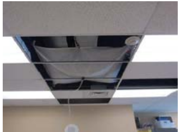
Figure A10.3.b – Ceiling leak
