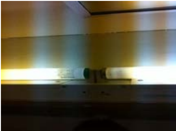
Figure D10.3.b – T12 lighting
