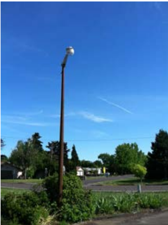
Figure E20.9 – Existing site lighting
