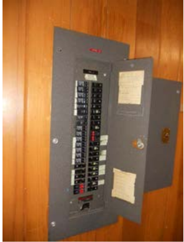
Figure D10.2.a – Lack of spare capacity
