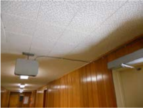
Figure D10.2.d – Door connected to lighting circuit
