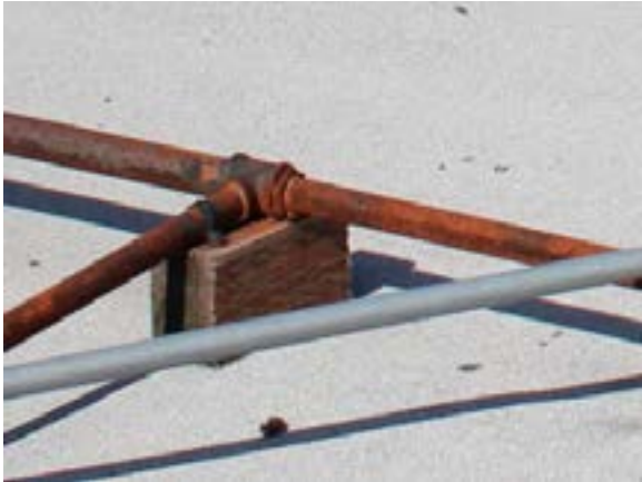
Figure C10.2.b – Gas piping corrosion
