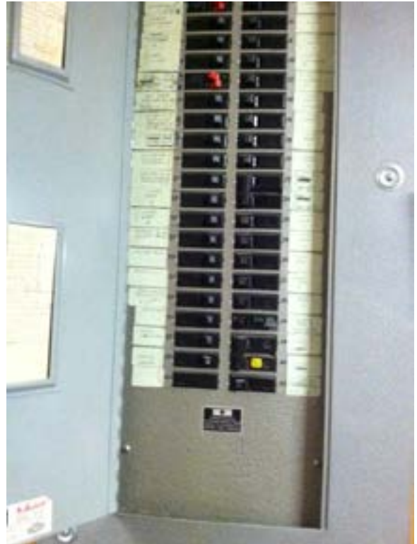
Figure D10.2.a – Lack of spare capacity
