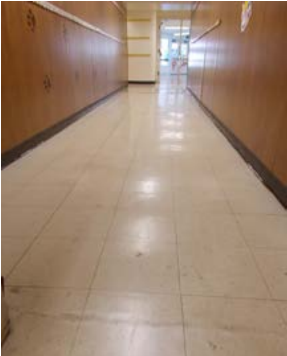
Figure B20.1.a – Flooring issues
