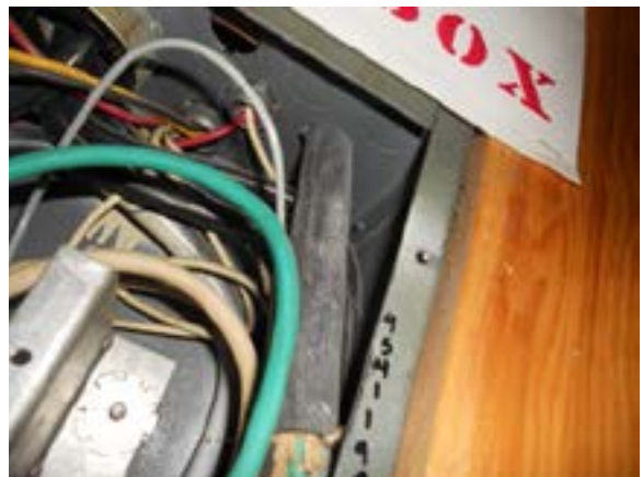
Figure D10.2.c – Wiring missing cable clamp
