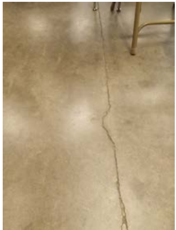
Figure B20.1.b – Flooring Issues
