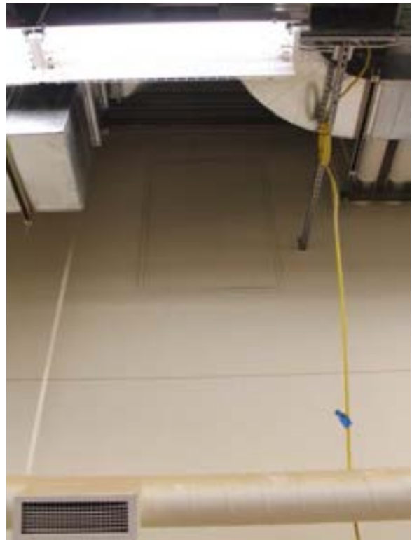
Figure C20.3 – Choir room ductwork access
