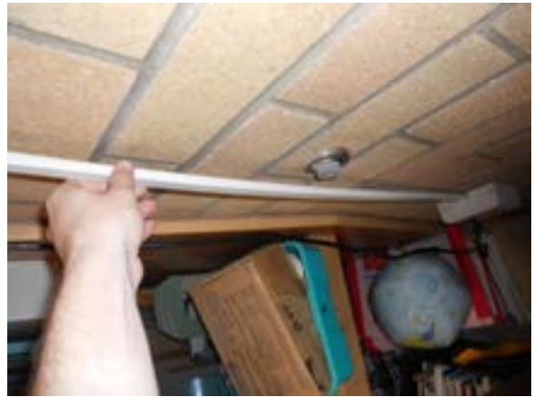
Figure D10.2.e – Wiremold missing fasteners
