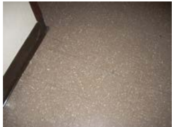
Figure B20.1.a – Flooring issues
