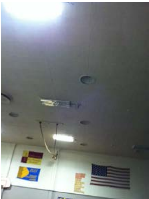
Figure D10.3.c – Hallways/Offices are overlit
