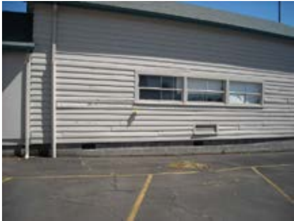
Figure A20.1 – Peeling siding
