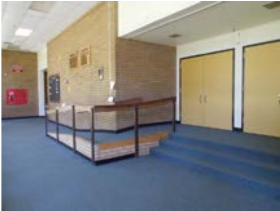
Figure B20.1.b – Flooring issues
