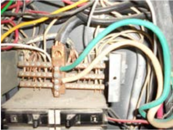
Figure D10.2.e – Overcrowded busbar
