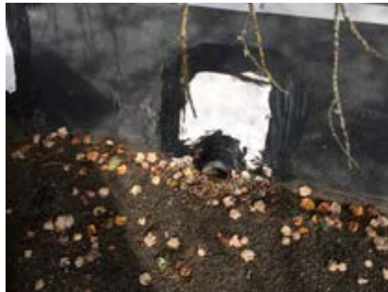
T-South Drain and EPDM wearing out
