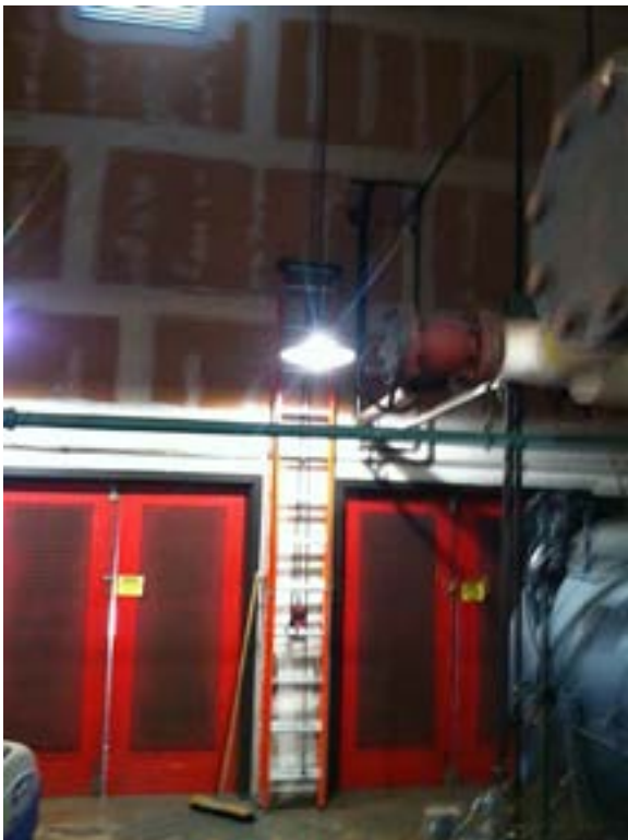
Figure D10.3.a – Mechanical room lighting
