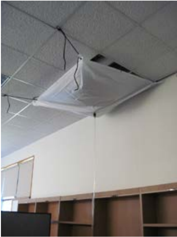
Figure A10.3 – Roof leak
