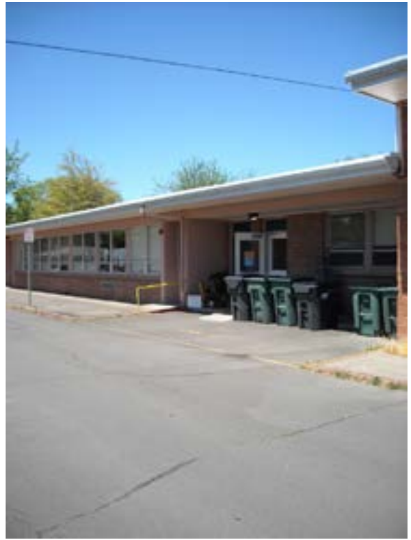
Figure E20.6 – Lack of trash enclosure
