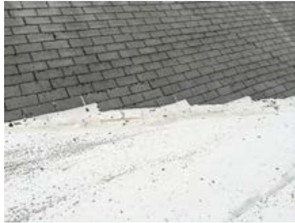
Shingles are brittle and falling apart
