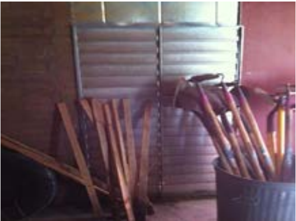
Figure D10.5 – Air louver blocked
