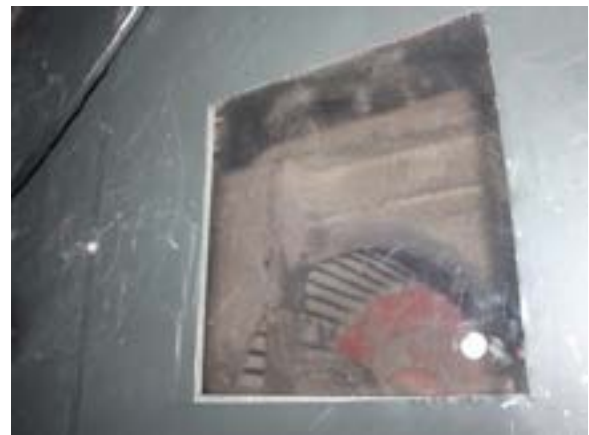
Figure C20.1.b – Dirty units from lack of accessibility
