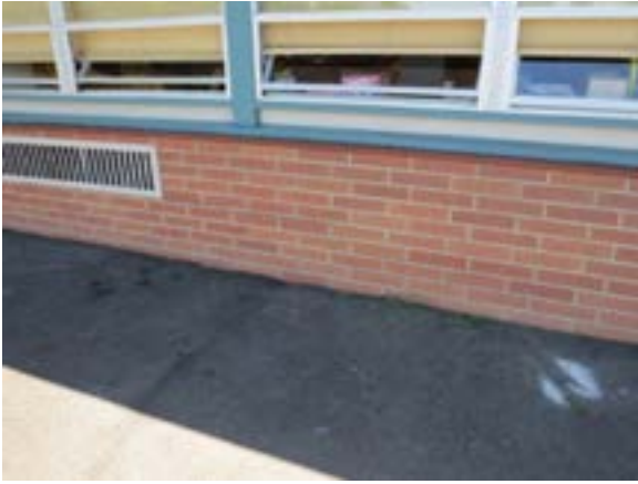
Figure A10.2 - Crack in masonry veneer
