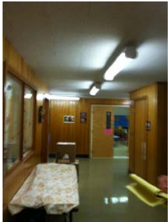
Figure D10.3 – Aging hallway lighting
