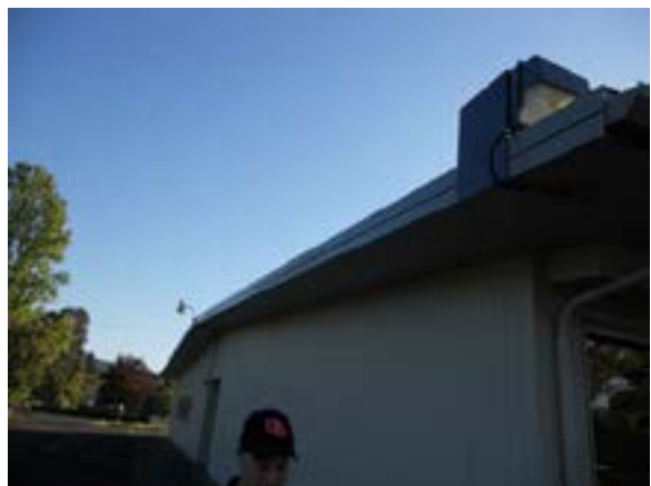
Figure E20.9.a – Insufficient parking area lighting
