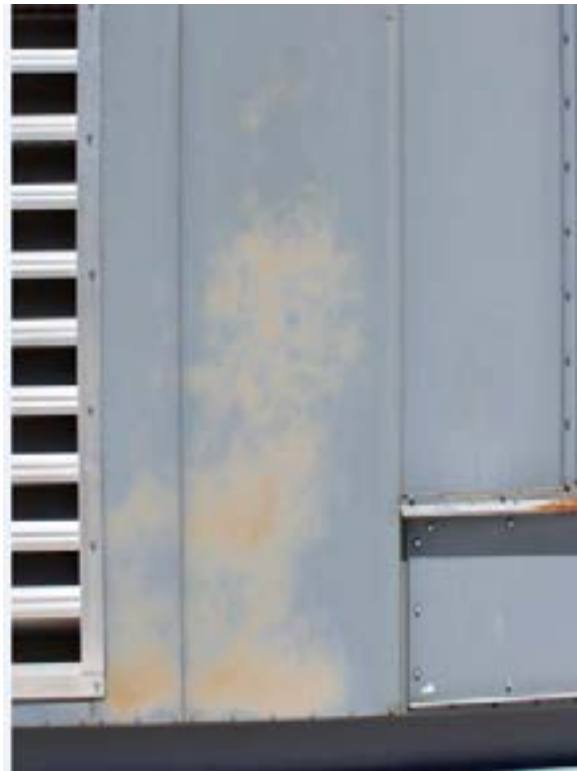
Figure C20.1.a – Paint failing on roof units
