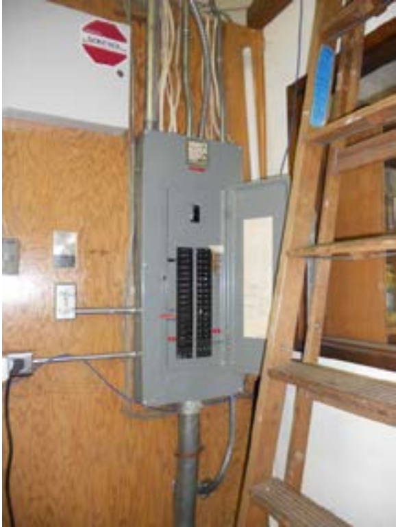
Figure D10.2.d – Existing electrical panel
