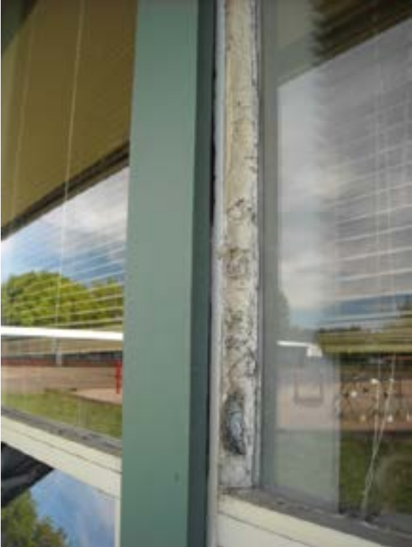
Figure A20.3 - Sealant Issues
