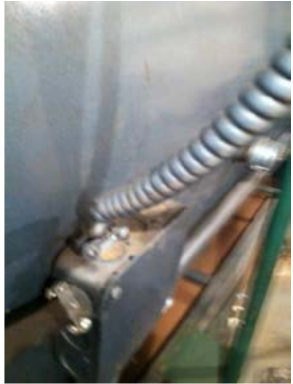
Figure D10.2.d – Damaged armored cable
