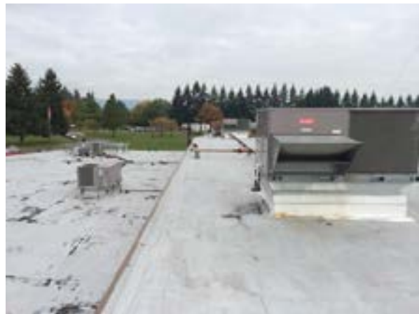
Emulsion wearing off, edges failing
