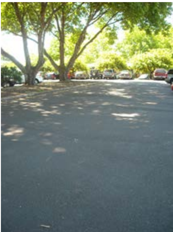
Figure E10.1.c – Tree root damage
