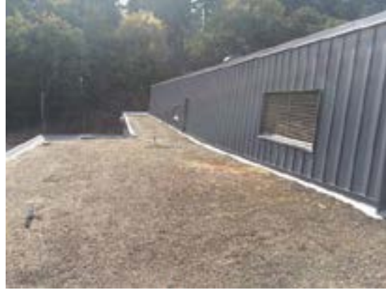
MOSS BUILDUP AT DRAINS AND MUST BE REMOVED
