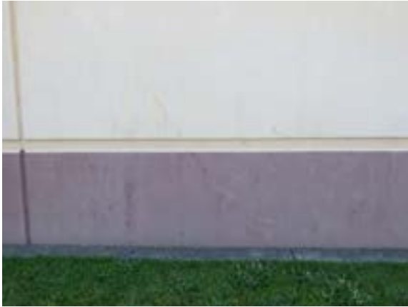
Figure A10.3.c – Cracks in concrete wall
