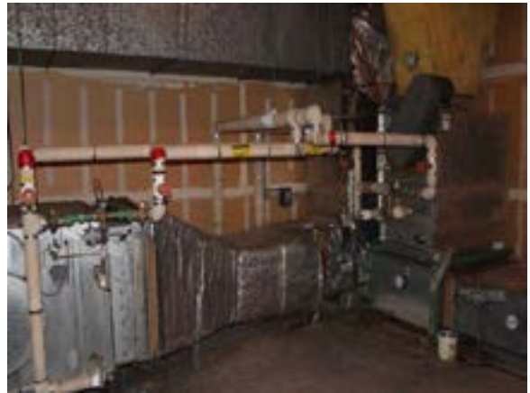
Figure C20.1 – Aging mechanical equipment
