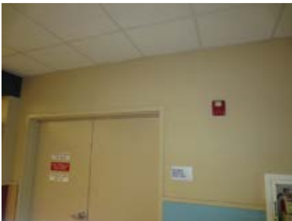
Figure A10.3.a – Crack in wall finishes
