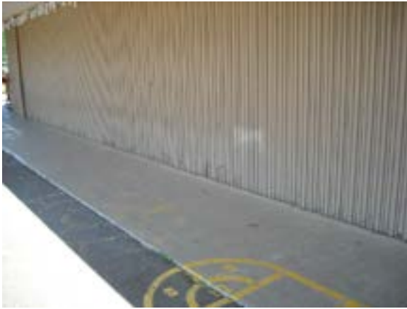
Figure A20.1 – Exterior wall damage
