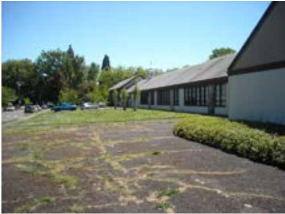
Figure E10.3 – Lack of parking
