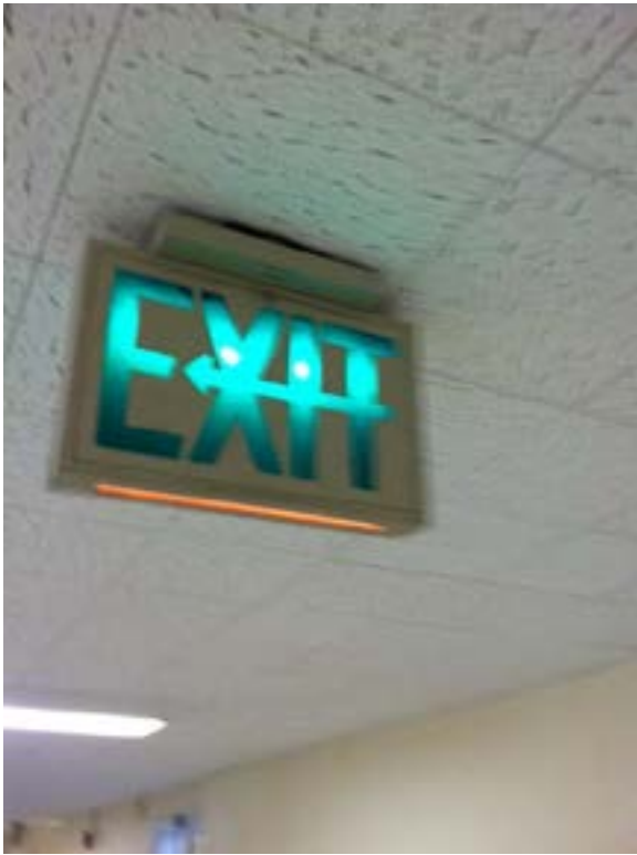
Figure D10.7 – Typical exit sign
