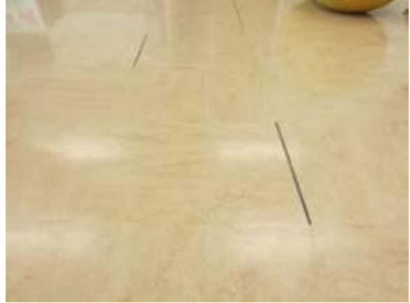
Figure A10.2.b – Slab on grade cracking
