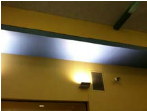
Figure D10.3 – Inadequate cafeteria lighting
