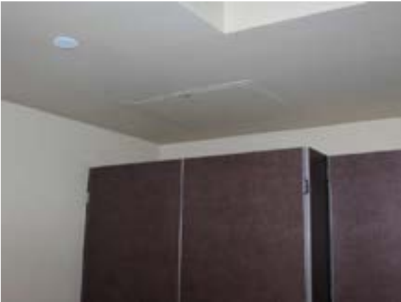
Figure C20.3 – Blocked fire/smoke damper
