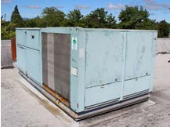
Figure C20.1 – Outdated mechanical equipment
