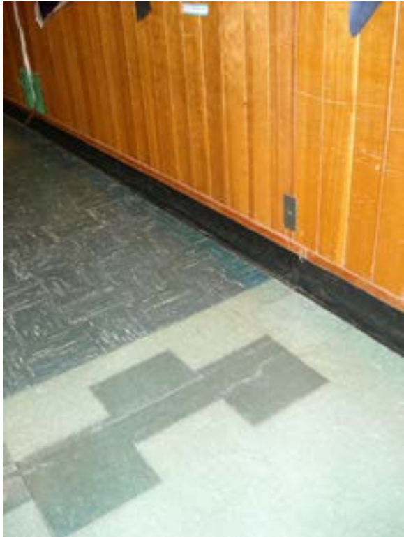
Figure B20.1.b – Cracks in hallway flooring
