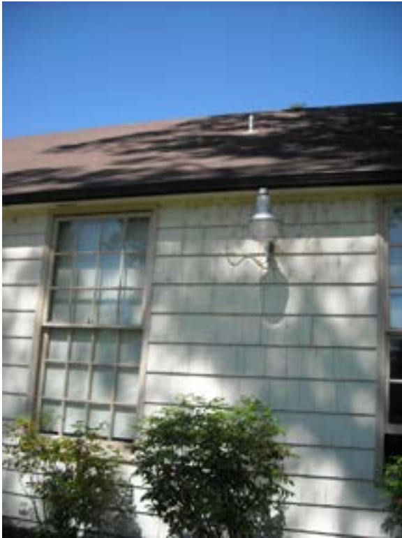
Figure A20.1 – Siding needs repainting
