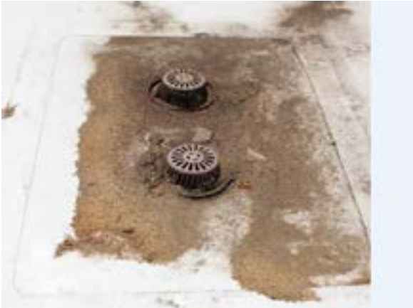
Figure C10.4 – Storm drains with sawdust
