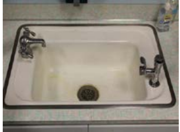
Figure C10.3 – Outdated plumbing fixture
