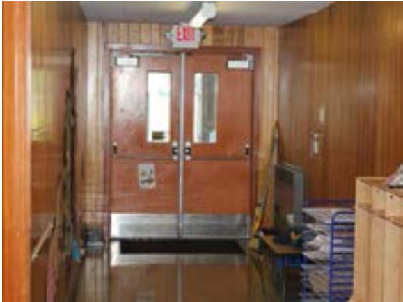
Figure D10.5 – Insufficient egress lighting
