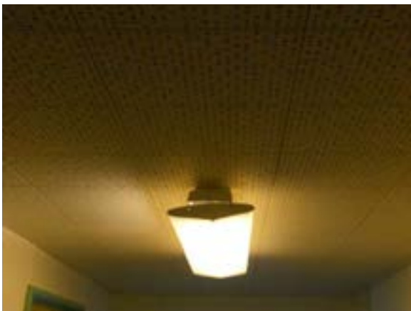
Figure D10.3.b – Dated hallway lighting
