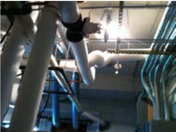
Figure D10.3.c – Mechanical room lighting
