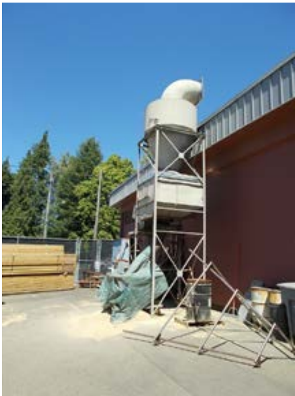
Figure B20.4 – Dust collector
