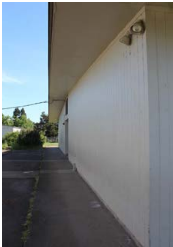
Figure E20.9.b – Incandescent site lighting
