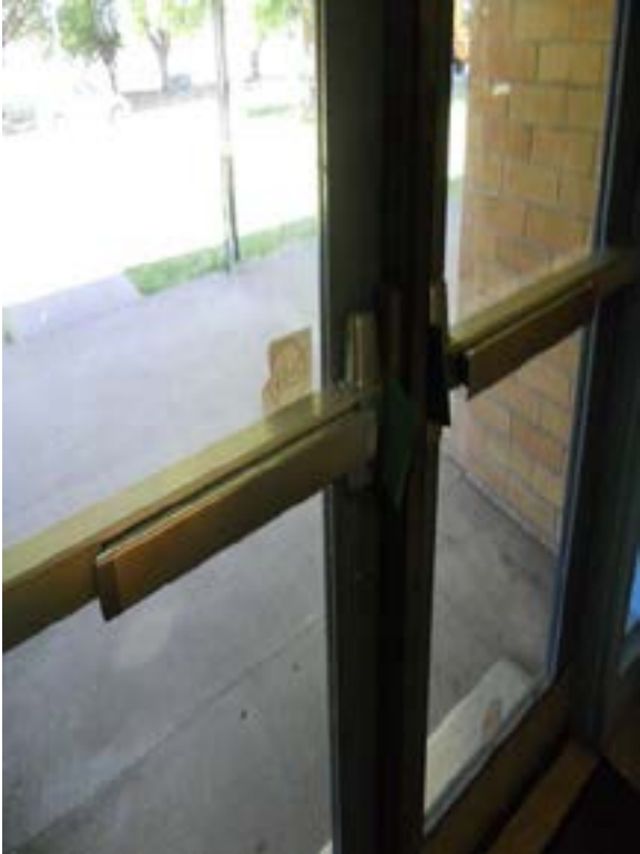
Figure D20.7 – Bypassed card access point
