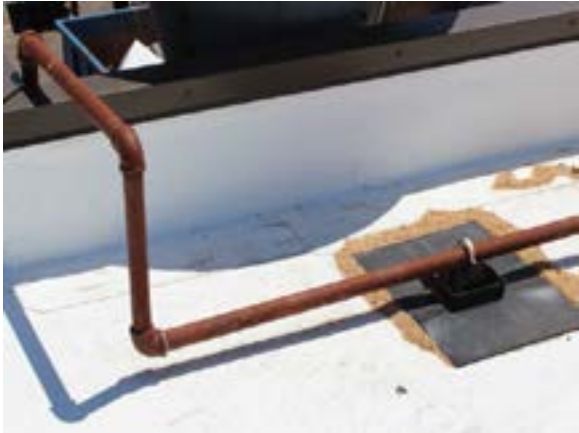
Figure C10.3 – Rusted gas piping
