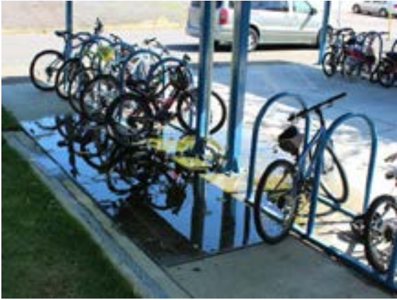
Figure C10.5 – Storm drain blockage
