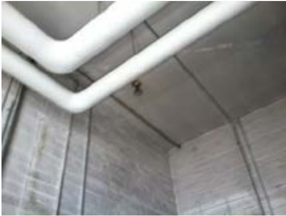
Figure D10.3.a – Mechanical room lighting
