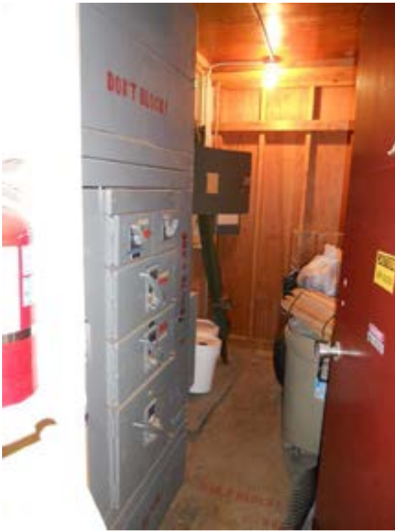
Figure D10.2.a – Electrical Room
