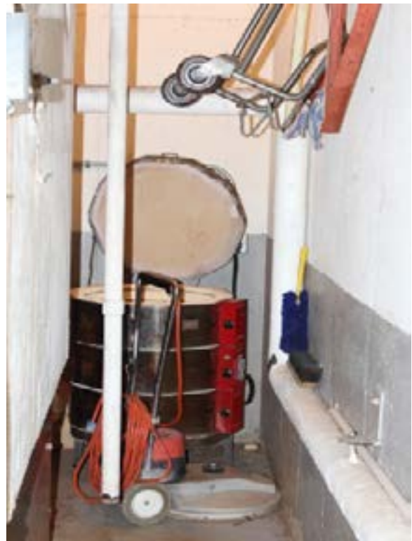
Figure C20.7.a – Kiln in boiler room
