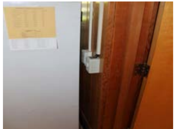
Figure C20.4 – Thermostat access blocked
