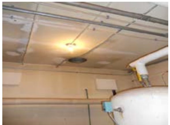
Figure D10.3.b – Mechanical room lighting
