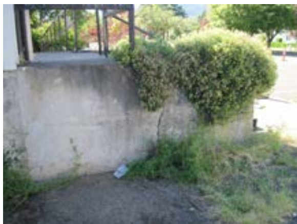
Figure A10.2 – Cracks in concrete wall
