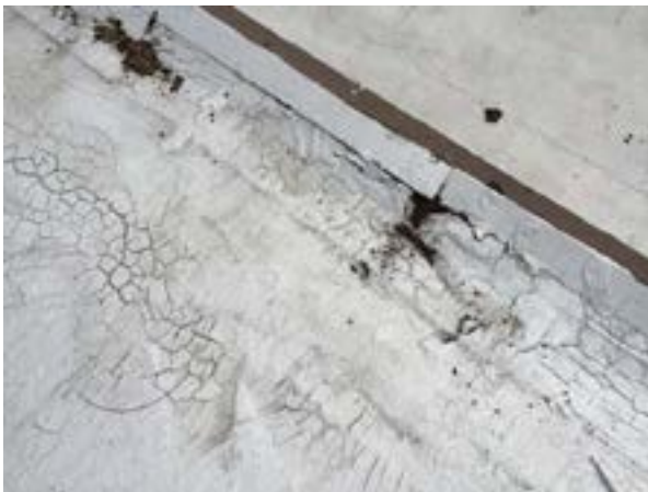
Cracking and Failing along edges of Roof
