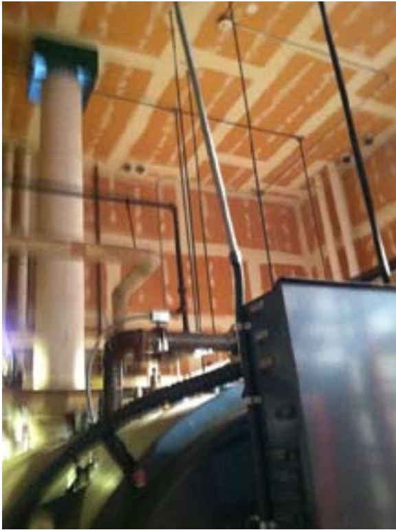
Figure D10.2.c – Incorrect conduit type
