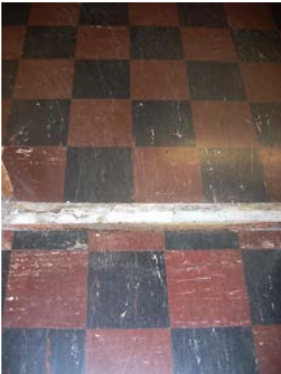
Figure B20.1 – Cracked flooring
