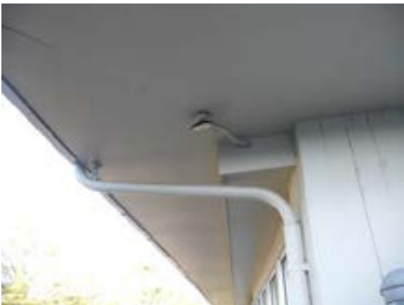
Figure D10.2.c – Junction box lacks cover
