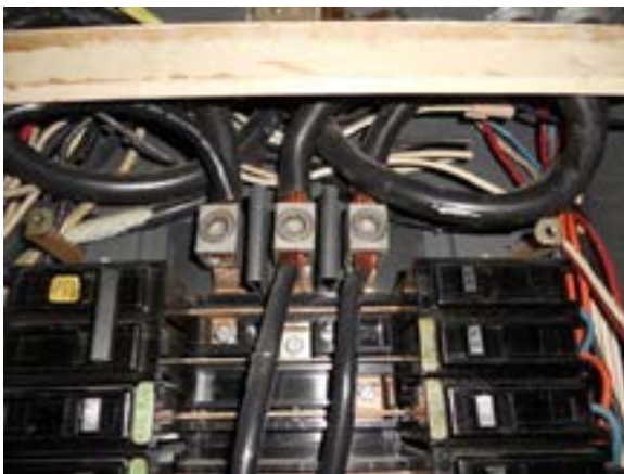
Figure D10.2.c – Existing branch panel conditions
