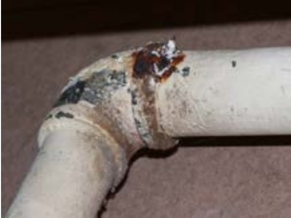
Figure C10.2.a – Sprinkler piping corrosion
