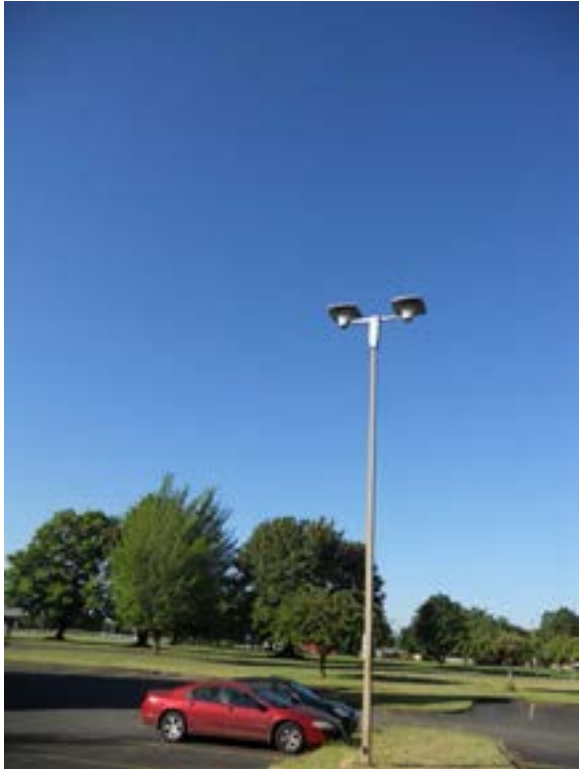
Figure E20.9 – Site lighting missing manhole cover
