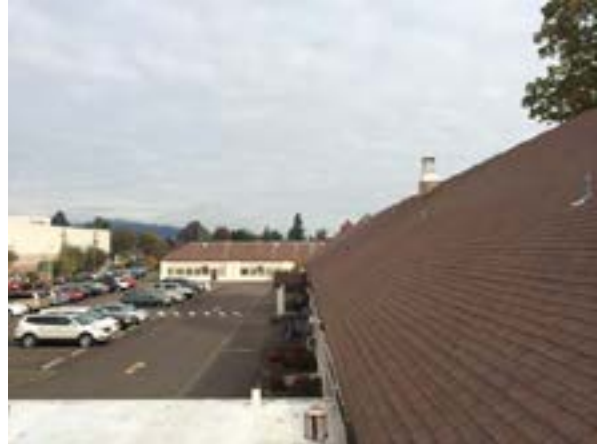
Shingles are brittle and breaking apart
