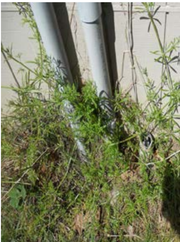
Figure D10.2 – Abandoned electrical feeder
