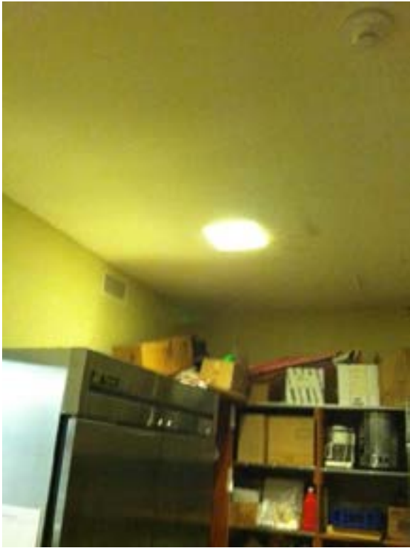
Figure D10.3.c – Kitchen lighting
