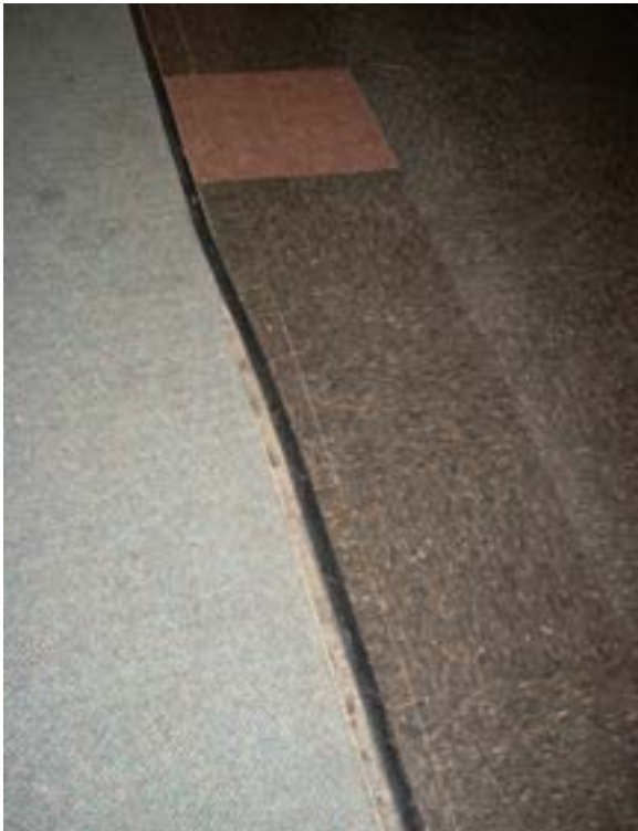
Figure B20.1.d – Flooring issues
