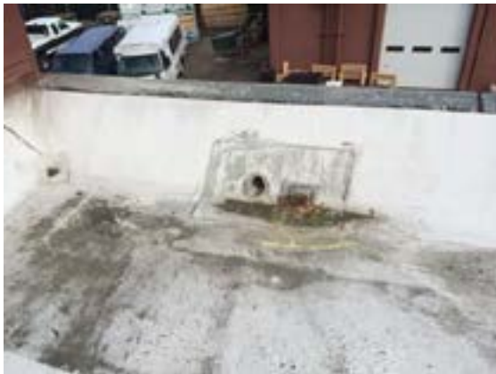
T-North Drain and TPO wearing out
