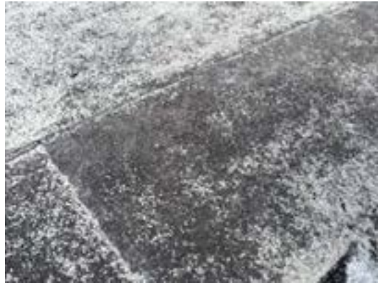
BUR WORN DOWN TO ASPHALT
