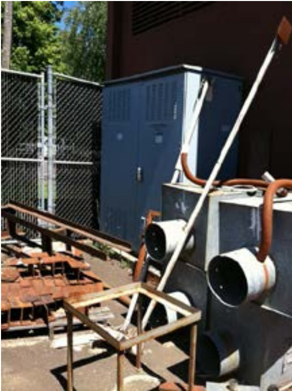
Figure D10.2.c – Inaccessible switchboard
