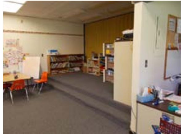
Figure B20.1.c – Flooring issues
