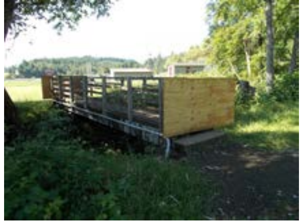
Figure E10.4.b – Condemned bridge
