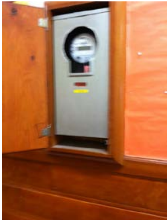
Figure D10.2.d – Noncompliant meter installation
