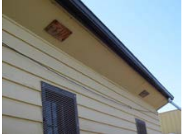
Figure A10.3 – Covered up roof vents
