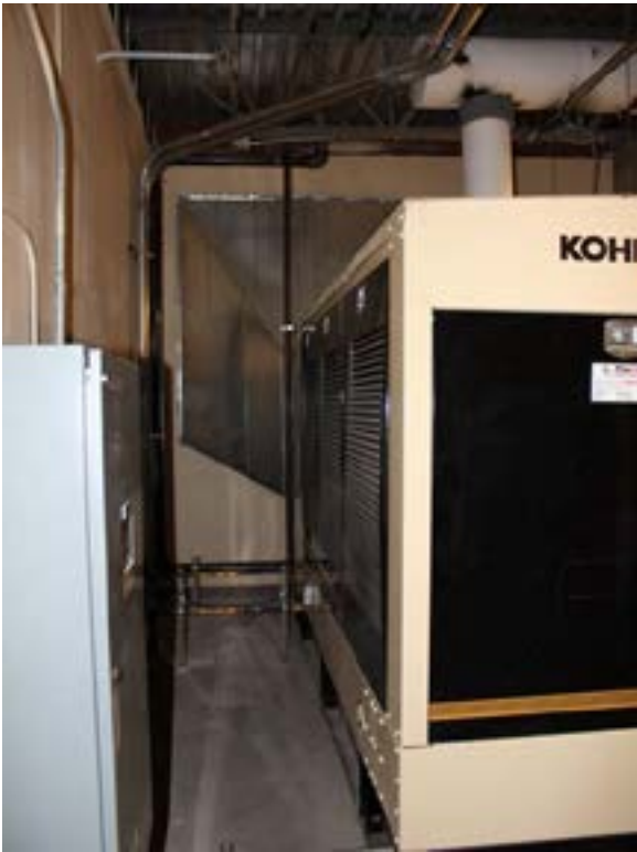
Figure D10.5.b – Insufficient space/access
