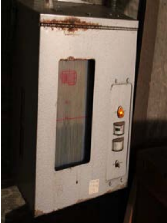
Figure D10.6 – Failed lighting inverter
