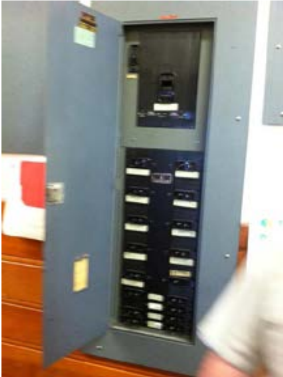
Figure D10.2.e – Panel lacks capacity
