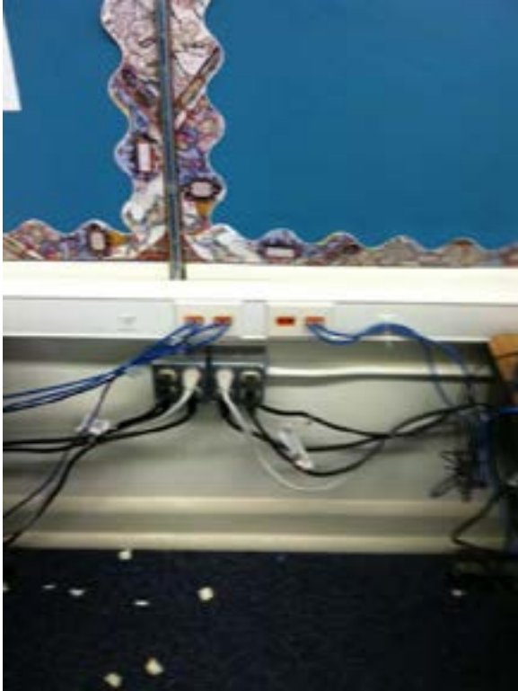
Figure D10.2.g – Insufficient classroom receptacles
