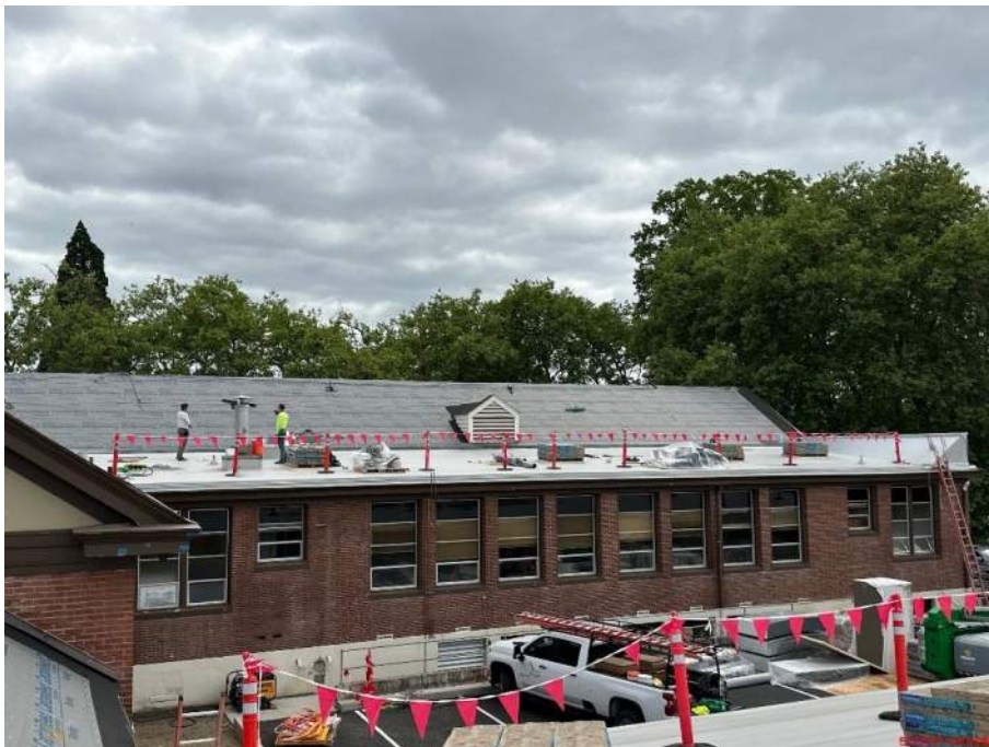
CHHS – New roofing going in on Area C roof (abatement of old flat roof complete)
