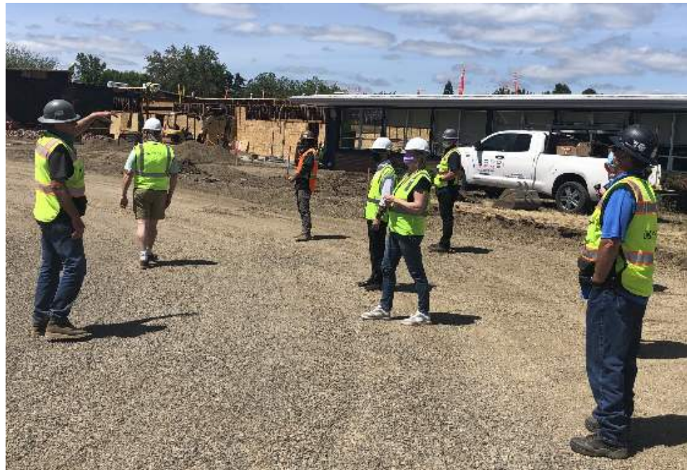
School board members being briefed by Fortis on the parking lot construction and the new office addition
