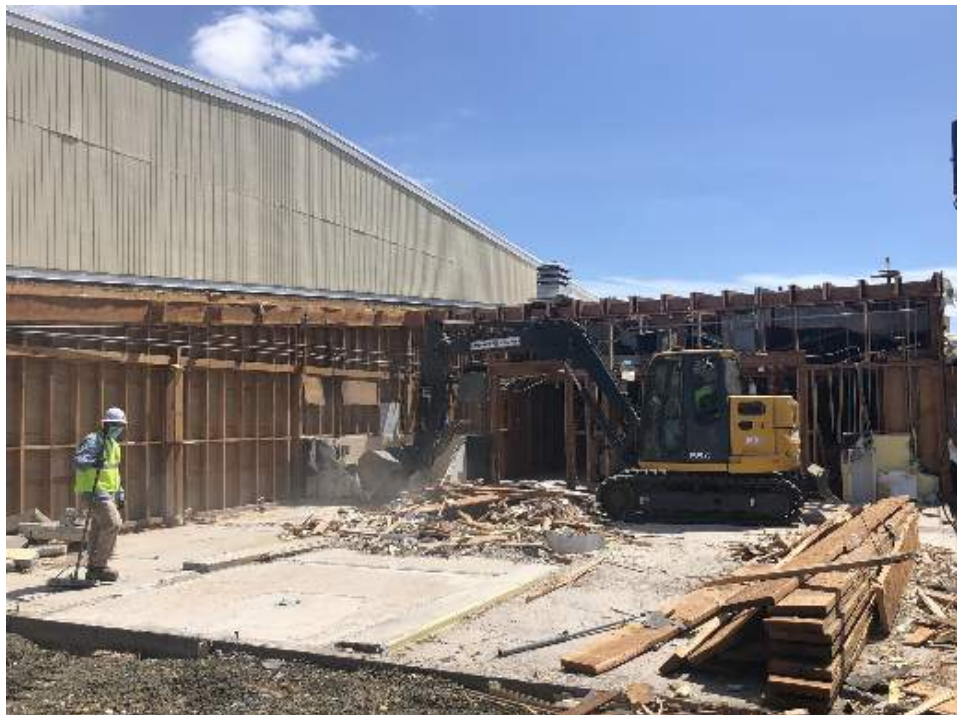
Old restroom and locker room area being demolished to make way for the new addition construction
