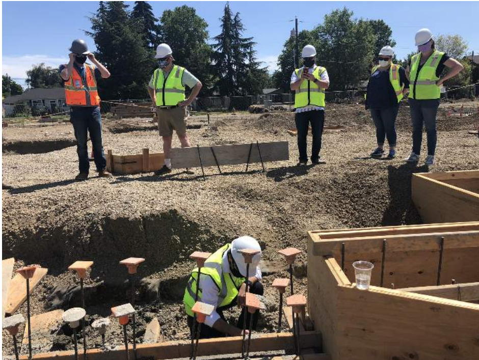
Board members inspecting the footings and carving their initials into wet concrete
